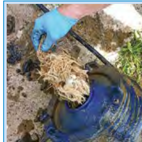
A CMSD maintenance worker disentangles wipes caught in a pump.
